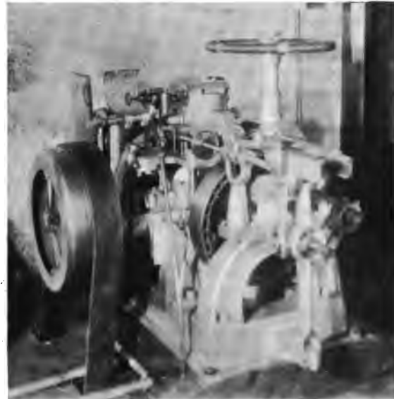
Fig. 4. Electric Controlling Device for Water Wheel.
